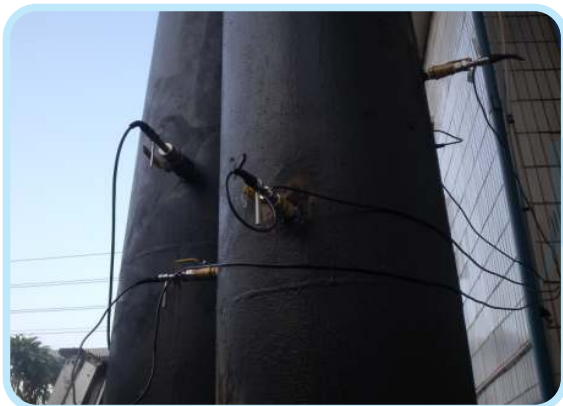
DN1000 Circulation Cooling Water
