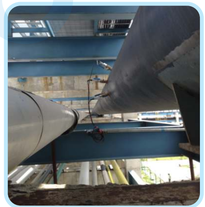
Power Plant Circulation Water
