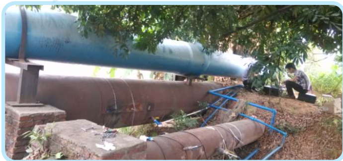
DN800 Water Supply
